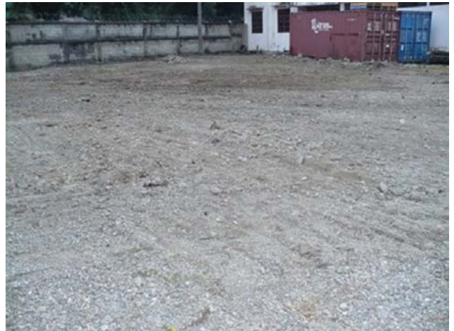
The site for the MMETM Education and Training Centre at Becora has been levelled in preparation for work to begin.
